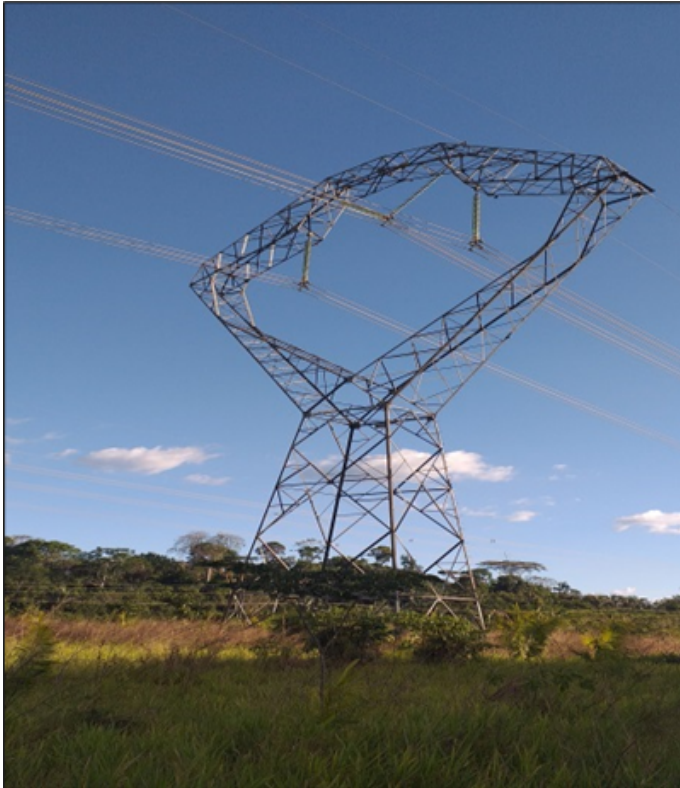
Figure 5.3: Power transmission towers.
