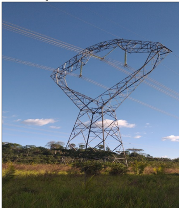
Figure 5.3: Power transmission towers.
